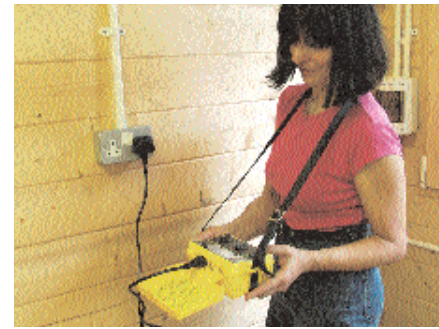
The trip speed of the RCD is measured. Test equipment is expensive, you must be trained to use it properly and it must be calibrated annually
