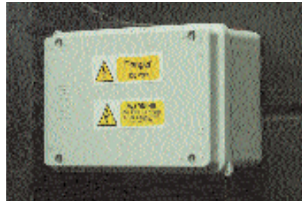
The connection to the workshop is made on the outside of the building and is housed in a weatherproof box which is labelled appropriately
