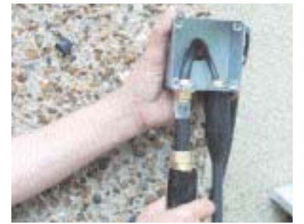
The switch and two-way lighting cables are terminated in an adaptable box. In a confined space it's much easier to fit the gland kits and armoured cables to the box before securing the box to the wall
