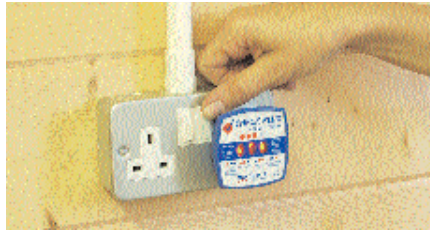
It is a requirement of the regulations that all work is inspected and tested. Some testing is done prior to connection. Here a simple plug-in tester is used to check that the connection to the sockets is correct
