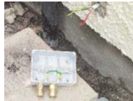
At the house end the connection is made in another weatherproof box. The armoured protective sheath is earthed to the main earth terminal at the consumer unit using a 6mm earth cable. This must be the same size as the phase conductor used to connect the consumer unit to the junction box to comply with the wiring regulations
