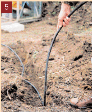
5 Dig a trench at least 450mm deep and lay the cable to the workshop
