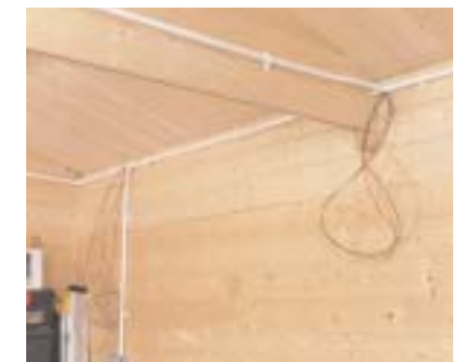
Work around the installation leaving loops at junctions to be pulled through once the end of the wiring has made it to the consumer unit
