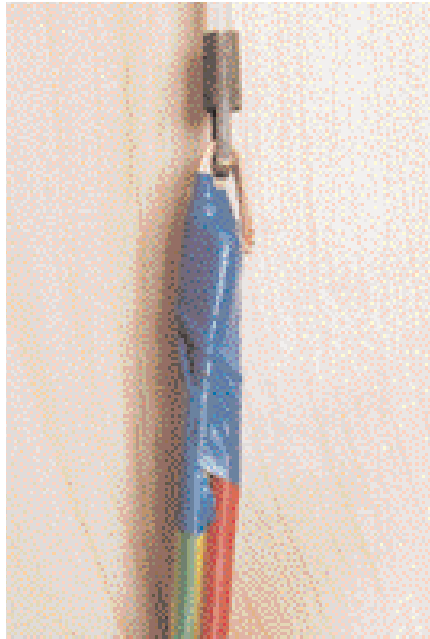
When it gets too hard to push the wire through it can be pulled through with a draw wire. Attach the wire and...
