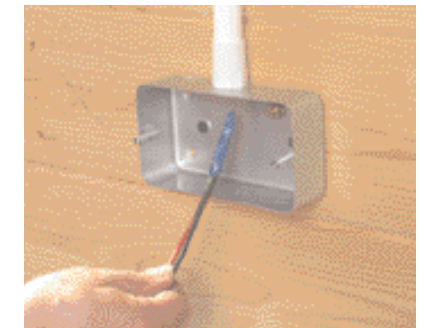
Run the wire from the furthest socket back to the consumer unit. Tape ends to make it easier to push through conduit
