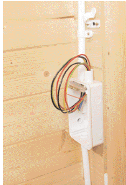
Back to the consumer unit and looped around to stop it being pulled back accidentally
