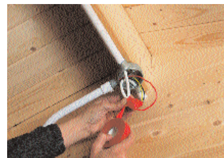
Connection is made between the single wire supply and the flex to the fittings at a screw terminal within the 'T' conduit box. This is taped after connection to maintain the correct level of electrical insulation
