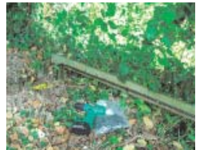
Here the switch cable is run back down to the house, fixed with plastic heavy duty clips. The incoming power cable will be fixed above
