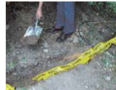
The buried cables have warning tape placed over them before the trench is back filled
