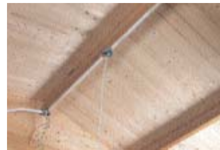
The conduit is threaded and screwed into metal conduit boxes. These are used to hang the fluorescent light fittings
