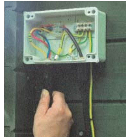
The cables are ready for connection to the shed. The armoured sheaths are being secured and connected to the workshop's main earthing block. An earth pole is fitted at the workshop. Although this is not strictly necessary it does ensure that the workshop has a good earth, regardless of what happens inside the house in the future. Box in the earth pole after installation
