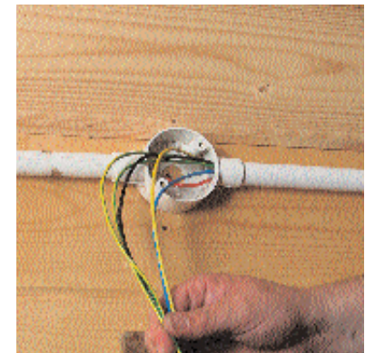
A hole is bored through the cabin to take the wiring for the outside light. Connection is made to the ring circuit
